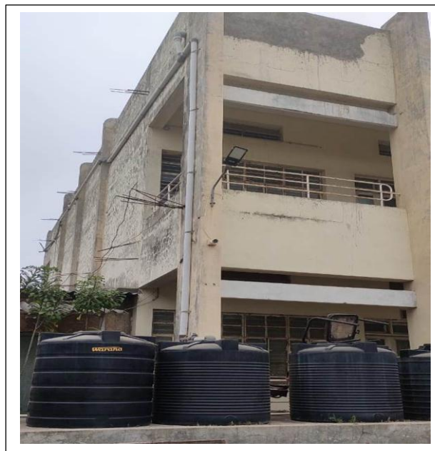
Rain Water Harvesting System
