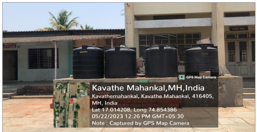
Rain water harvesting facility in the premises
