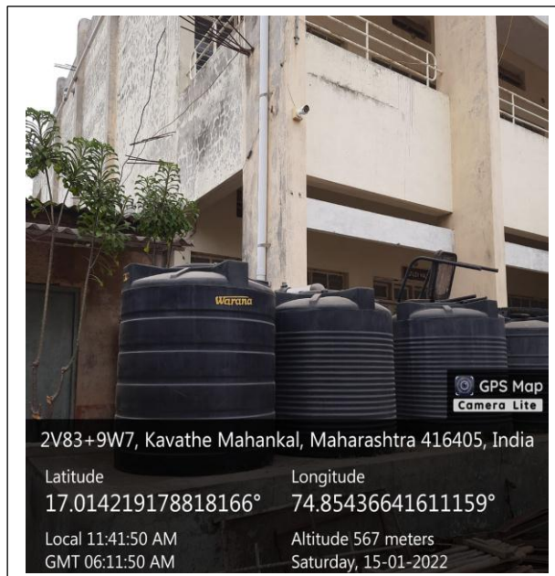
Rain Water Harvesting System
